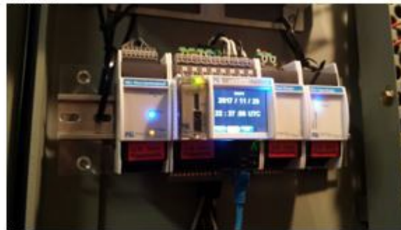
Figure 4: microPMU with GPS synchronized timestamps installed at Generator substation at IFP
